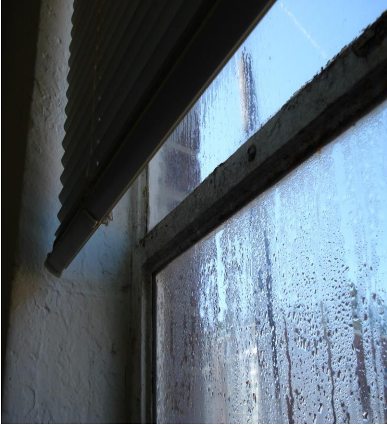
Condensation on cold window
